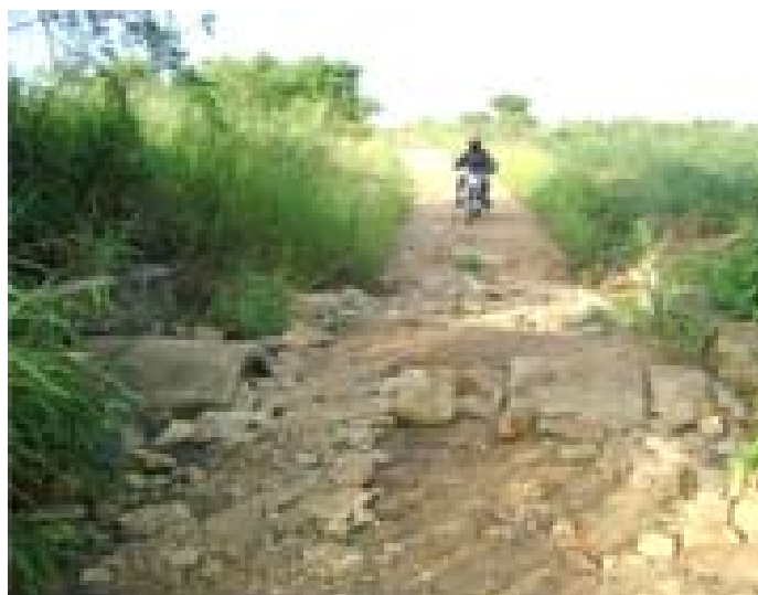
Figure5: Inaccessible road to Paminya Health Center-Nyaravur sub-county
