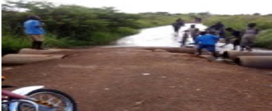
Figure 6: A section of Barotiba road in Patongo Sub-county, Agago District cut off by rain water
