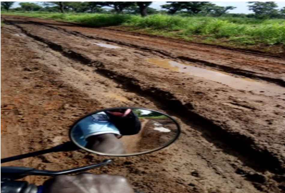
Figure 5: Geregere Okol road, Nakapiripirit District showing a poor road surface
