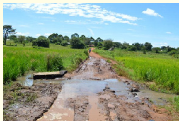
Figure 3: Poor quality works in swampy areas renders them impassable during the rainy season
